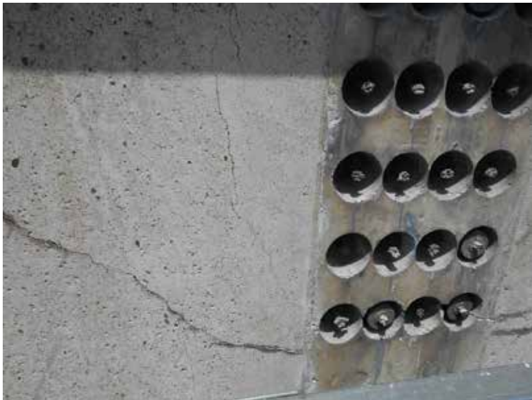
Fig. 8: Shear cracking at post-tensioned cable anchorage
