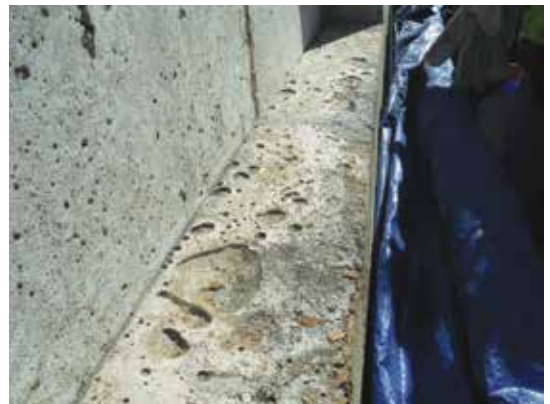
Fig. 3: Honeycombing damage on concrete beams
